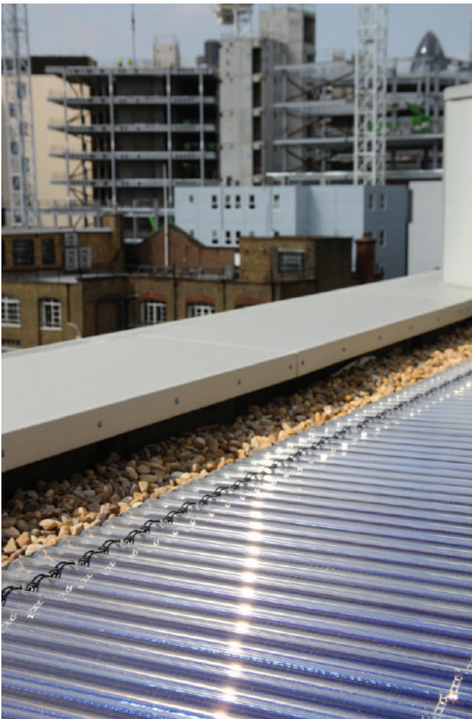
Solar thermal tubes for pre-heating of hot water
