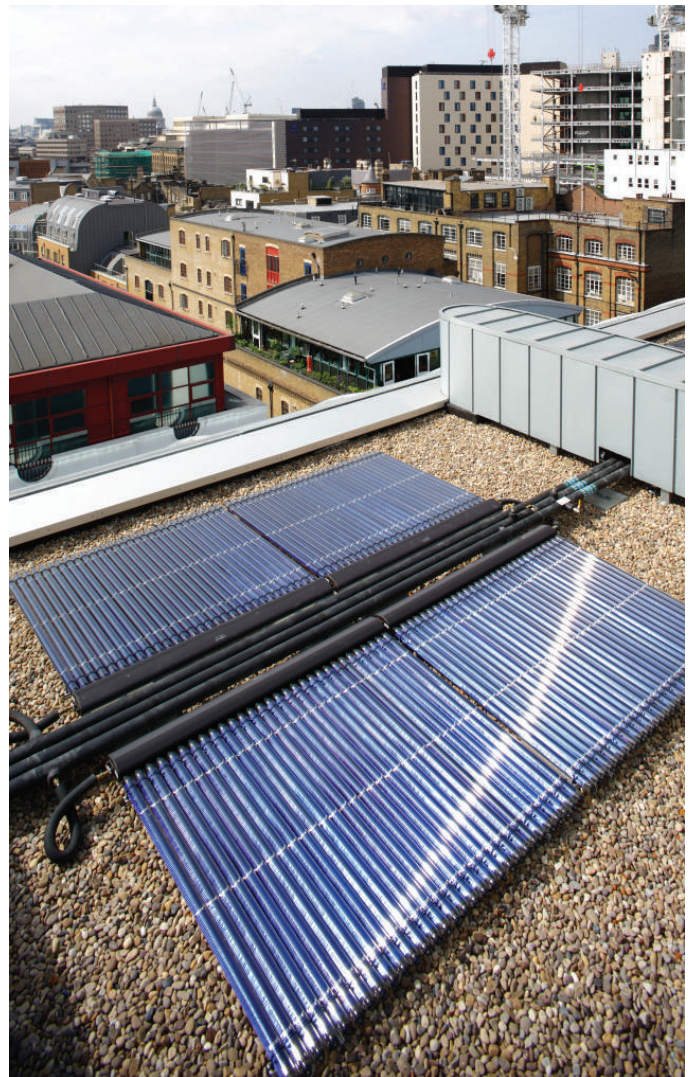
Solar thermal tubes
