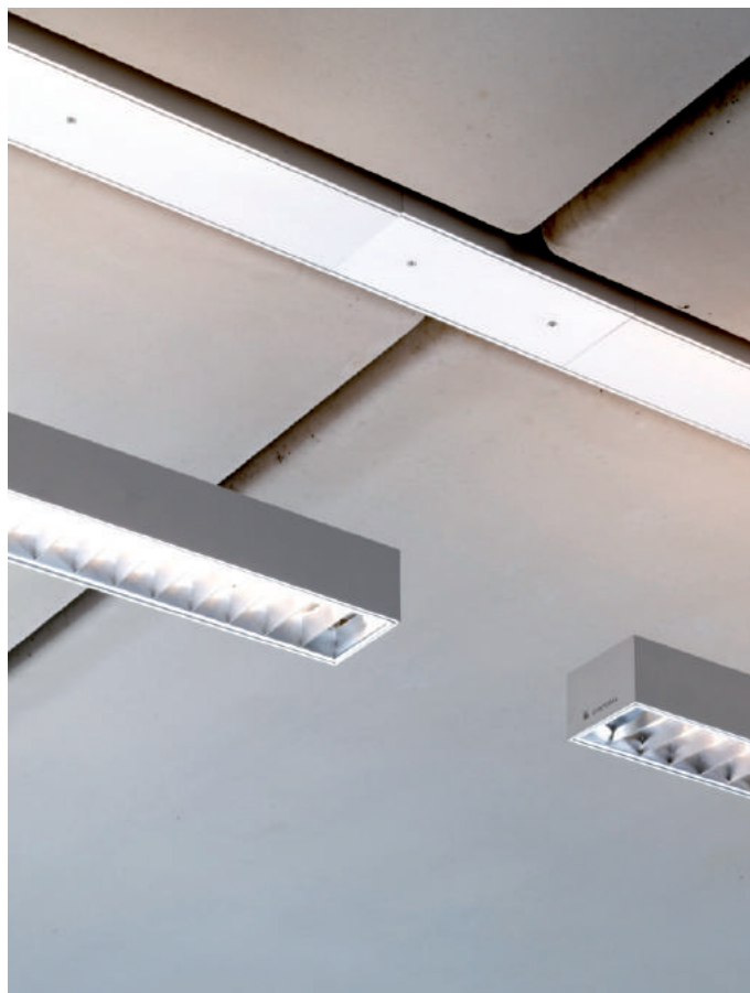
Soffit panels with integrated services and bespoke lighting
