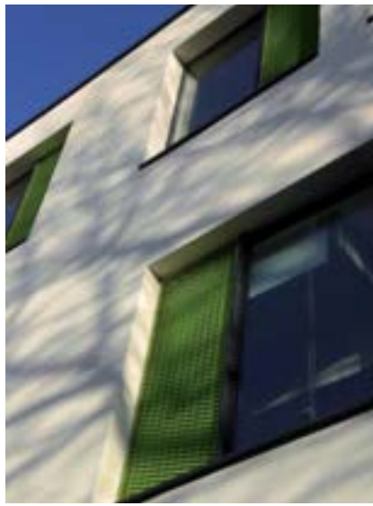
Opening casement windows that enables night time cooling
